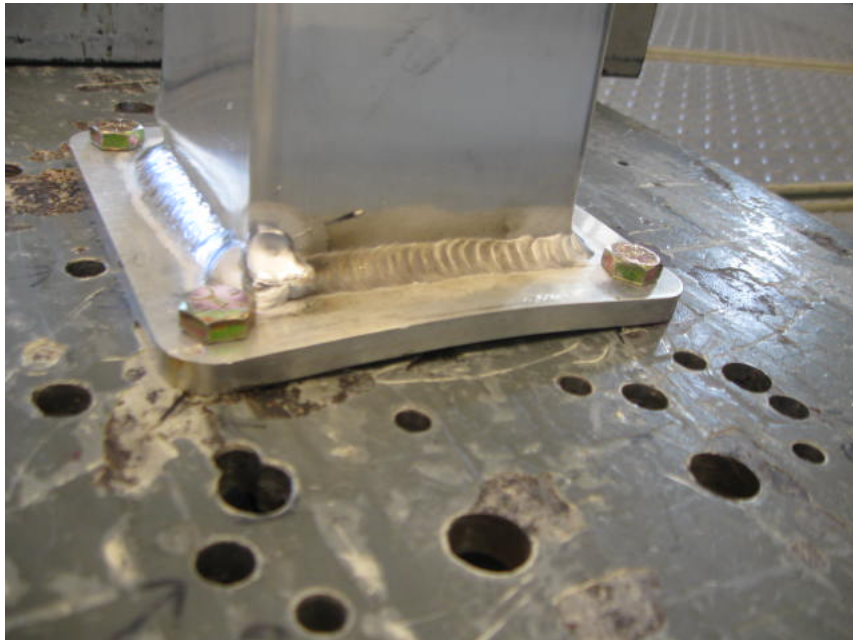
Photo No. 2 Typical base plate deflection under load
